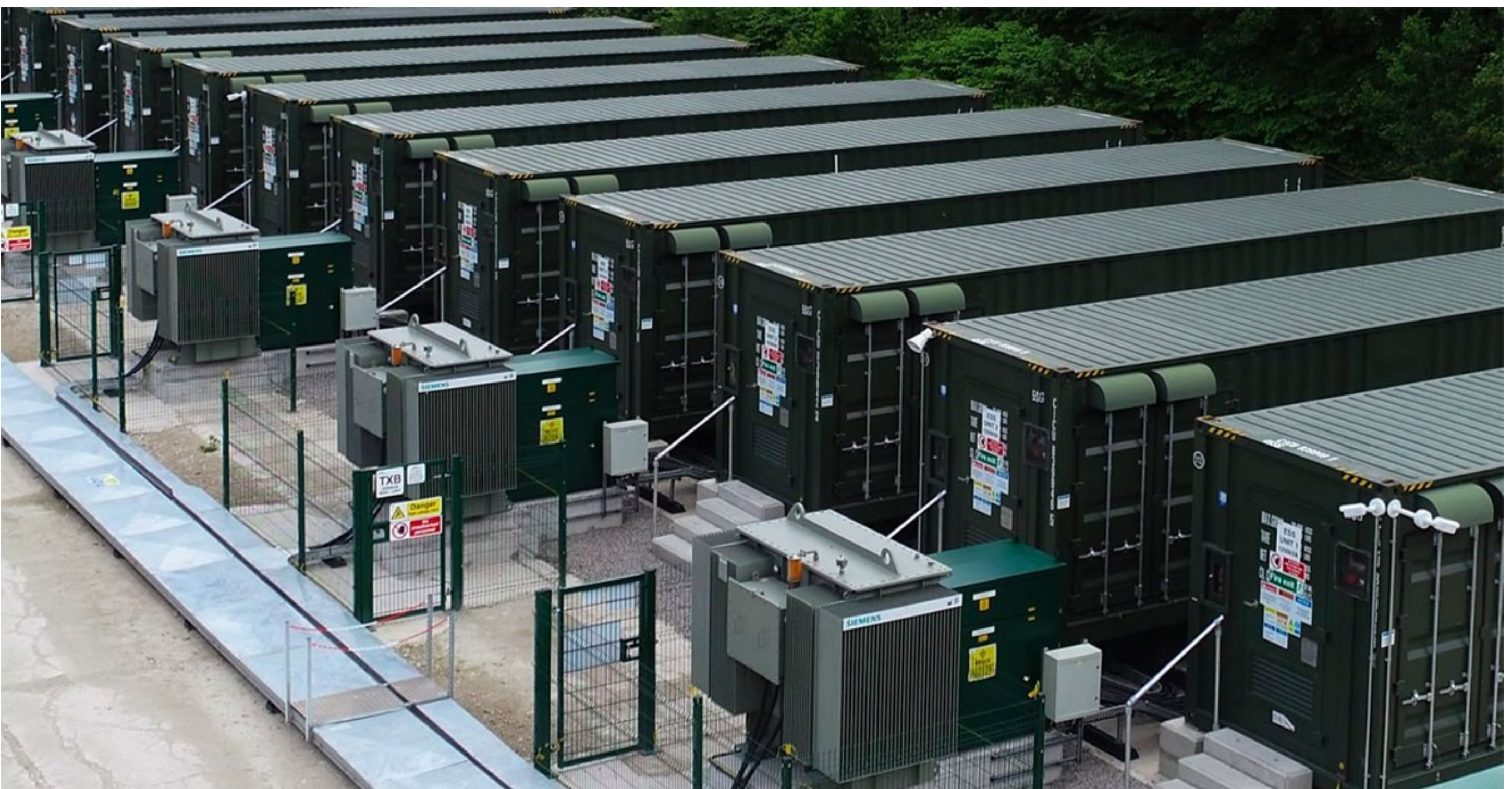
Illustration 6 : Typical Image of BESS Equipment : Source: www.jpsil.co.uk/
