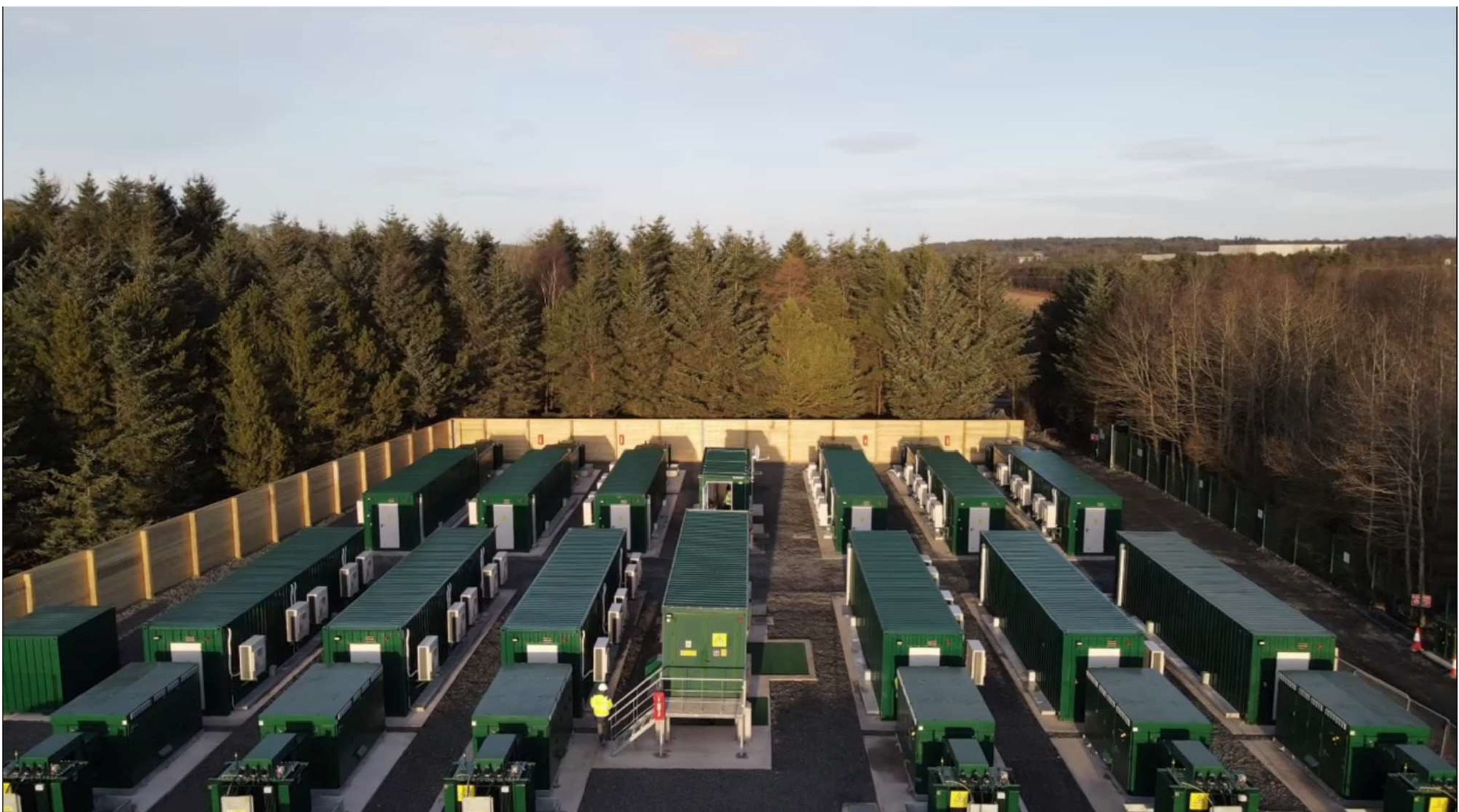
Illustration 5 : BESS Facility at Braes Brae, Scotland
